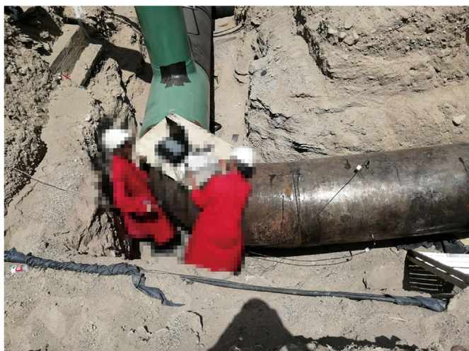
Fig. 2. Field condition of tested pipe section.
